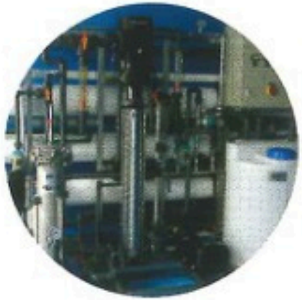
GENERAL PURPOSE WATER TREATMENT
