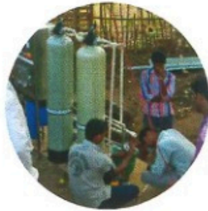
RURAL DRINKING WATER PURIFICATION PLANTS
