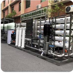
Pre-Treatment Before RO
